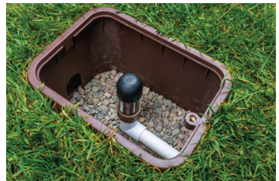
Air/Vacuum Relief Valve Installed
